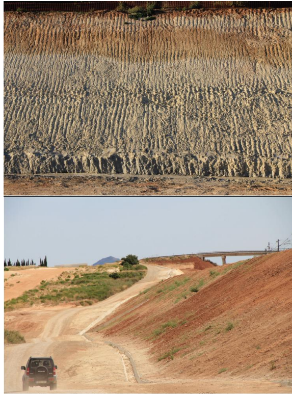
Figure 4. Photographs of the road and railway embankments studied. Note the lack of vegetation cover in both photographs and prominent rill development in the upper photograph.
