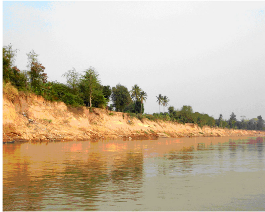
Fig. 10. Photographs showing streambank erosion along the Lower Mekong River in Vientiane, Laos. 2325
